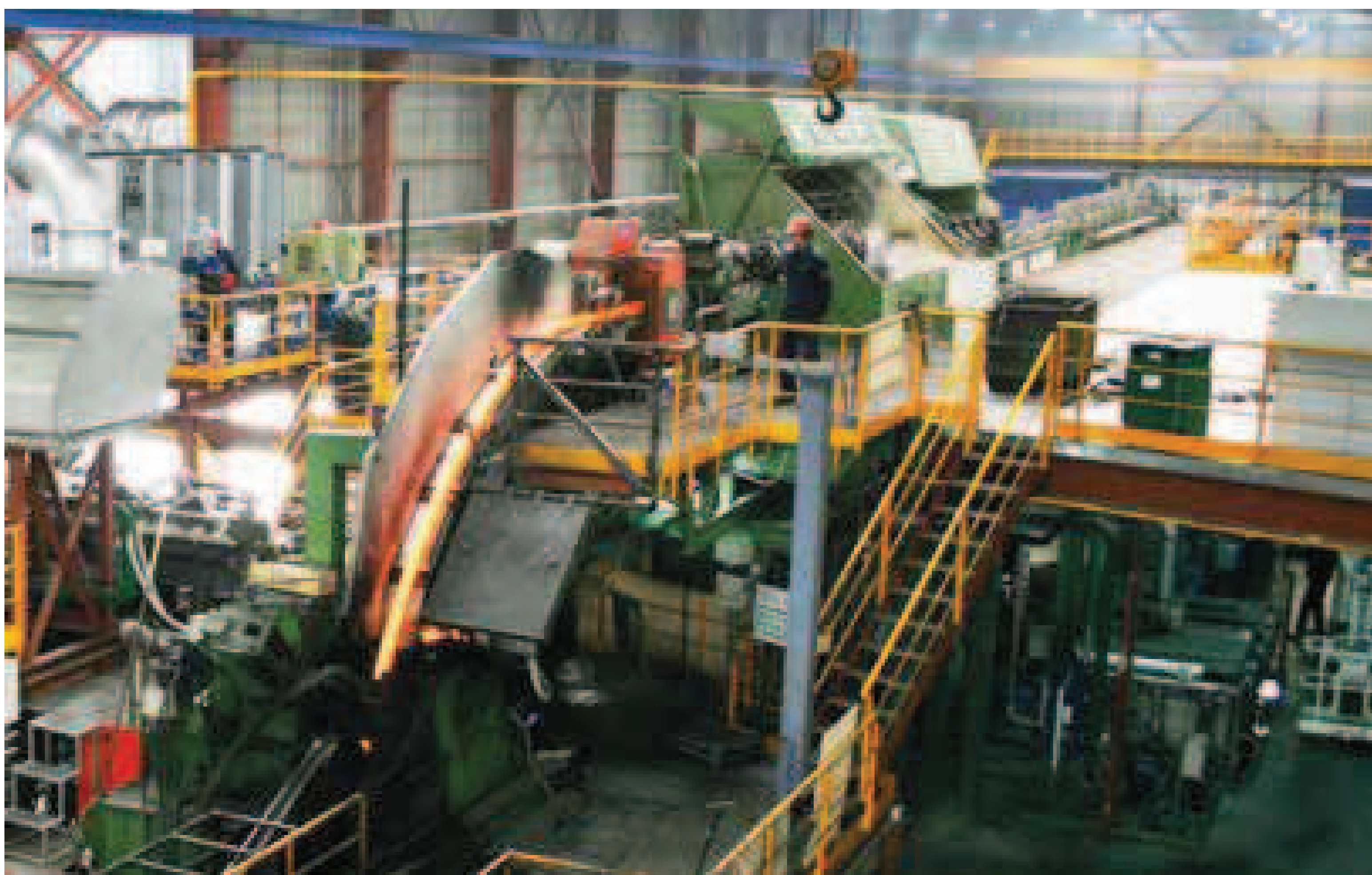
25 tph copper rod plant.
