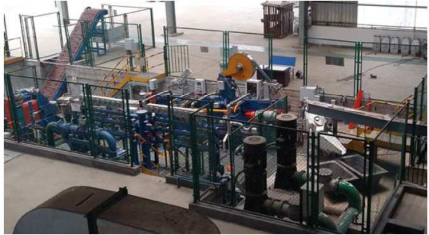
Figure 1. A Properzi track and belt caster in operation. Using closed-top molds, the caster is able to reduce the carbon footprint of the process.
