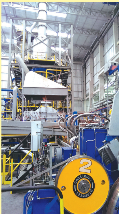
Shaft & Holding Furnaces of a CCR CU Line.
