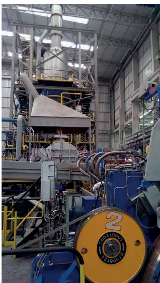
Example of Properzi Shaft and Holding Furnaces
